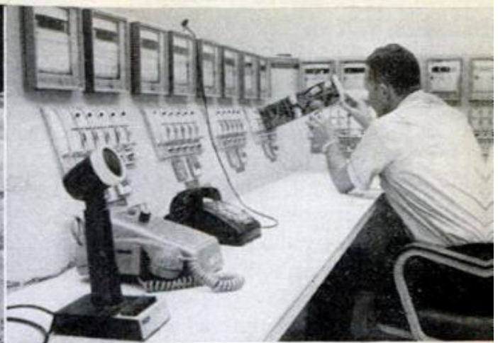
CENTRAL ENERGY PLANT provides power, airconditioning and water; uses natural gas to cut down on pollutants. Engineer at the control board monitors complex operation
